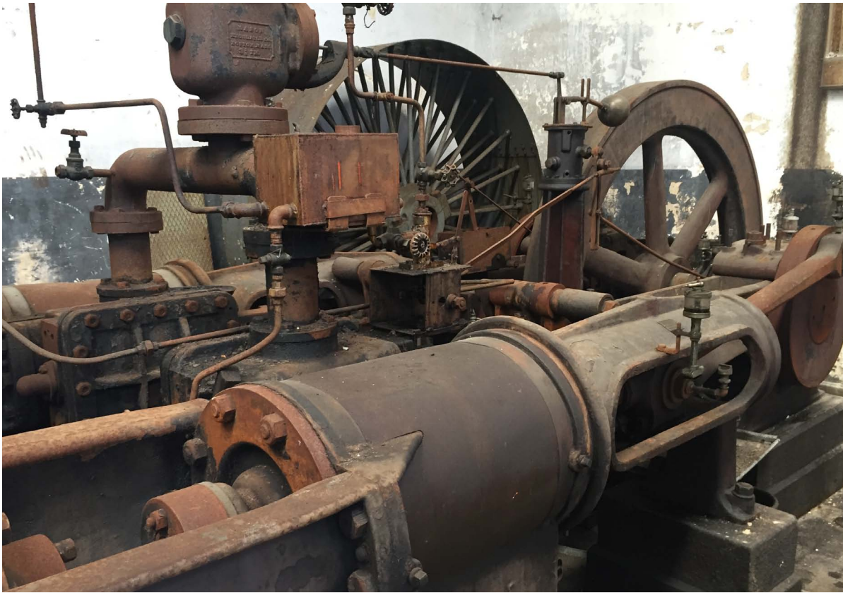
One of the horizontal steam engines in the power hall.
